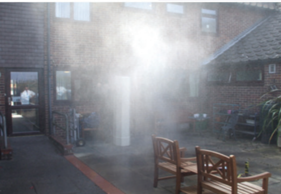
Sprinkler in action controlling fire spread
