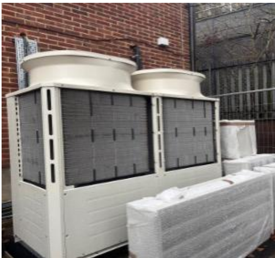
Caversham Road Fire Station – Air Source Heat Pumps
